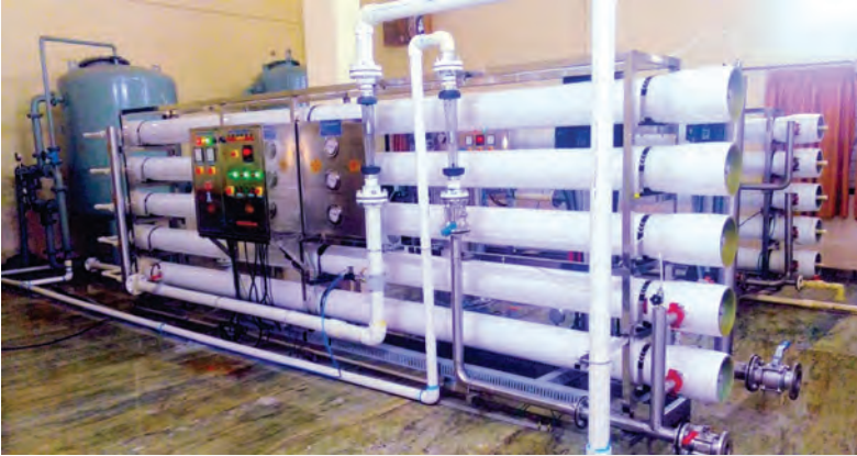
50 M 3 hr Reverse Osmosis Plant Installed in Logistic Park, Hyderabad
