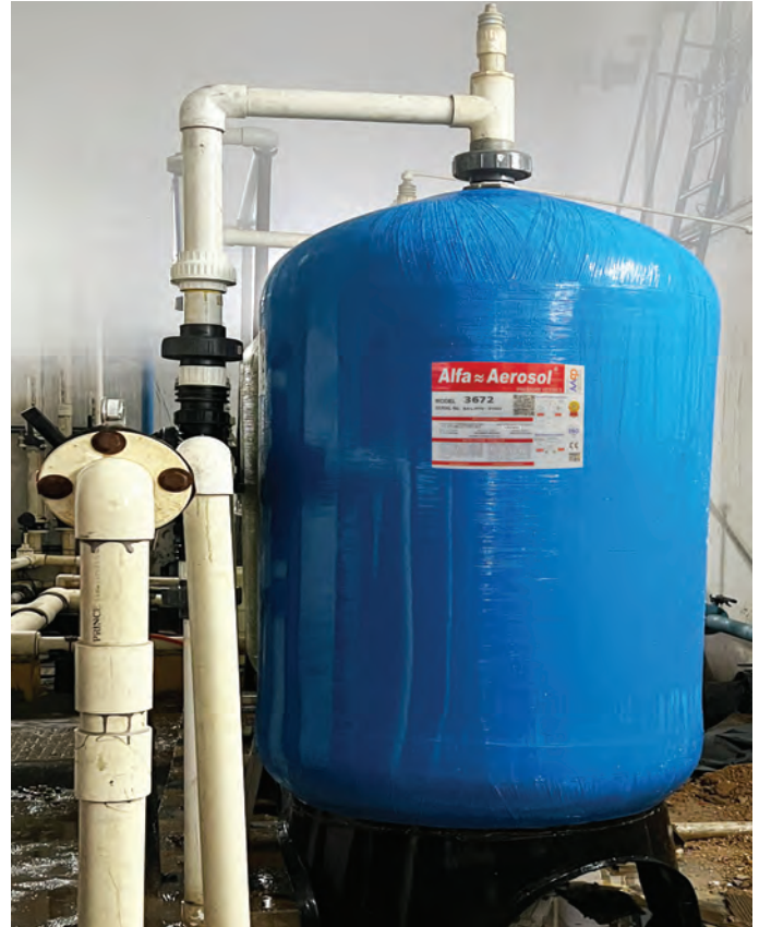
3672 FRP Pressure Vessel for Industrial RO Water Purification System installed in Le-Meridien
