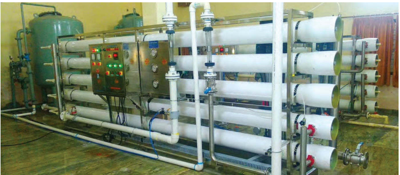
50 M 3 hr Reverse Osmosis Plant Installed in Logistic Park, Hyderabad
