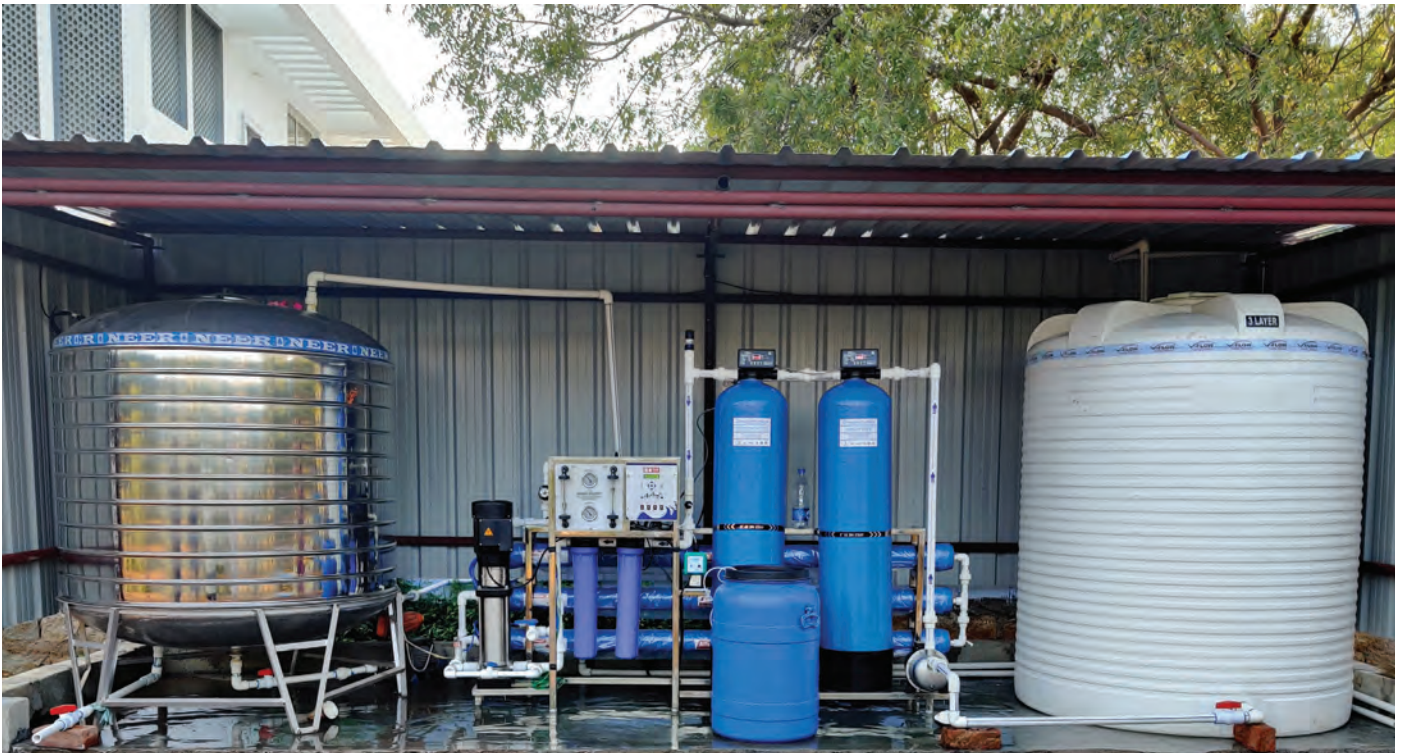
24 KLD Fully Automatic RO Water Treatment Plant
