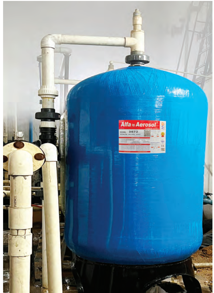
3672 FRP Pressure Vessel for Industrial RO Water Purification System installed in Le-Meridien
