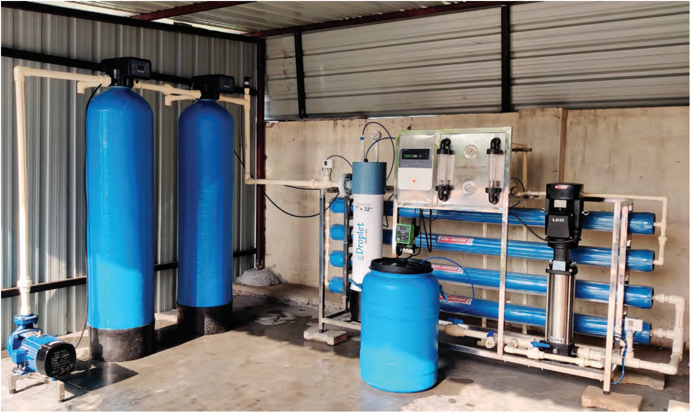
2000 LPH Fully Automatic RO Water Treatment Plant
