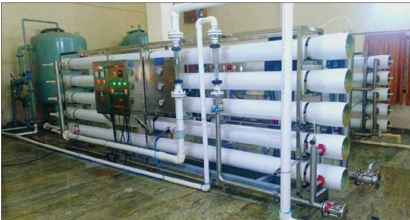
50 M3 hr Reverse Osmosis Plant Installed in Logistic Park, Hyderabad
