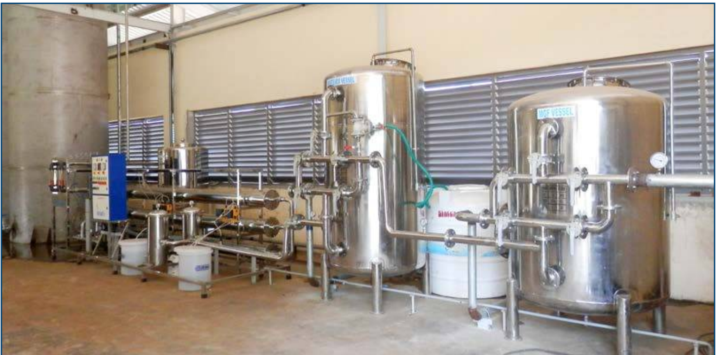
600 KLD Reverse Osmosis System for Boiler Feed
