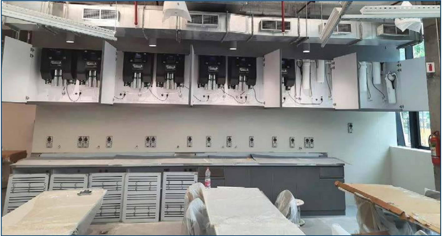
600 GPD Water Treatment & Storage Plant at Facebook India, Gurgaon
