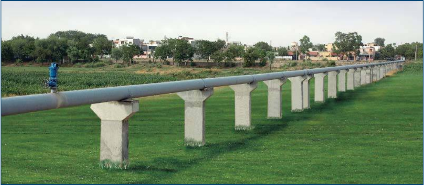
Bisalpur Jaipur Water Supply Pipeline
