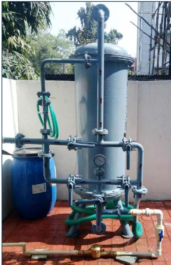
30 KLD Water Treatment Plant by Aquality Water Solutions
