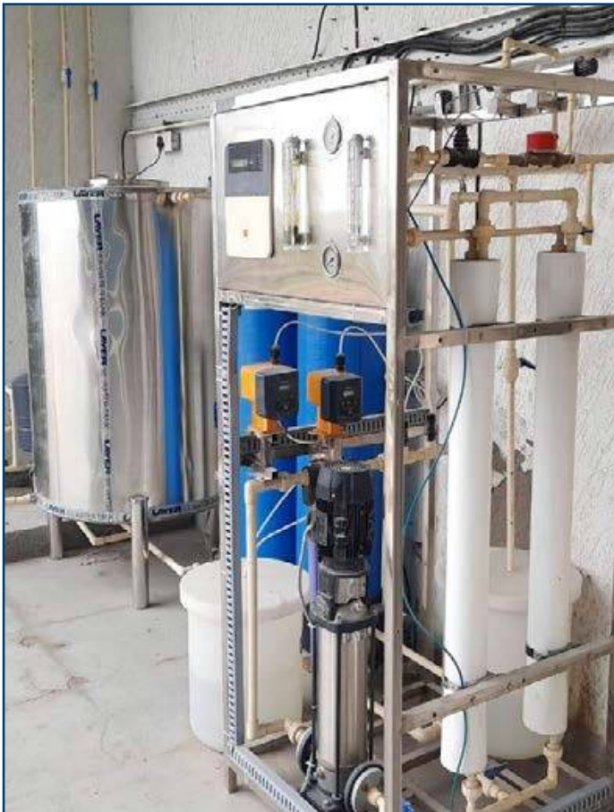
4000 LPD 6 stage Drinking water plant for Amazon Campus, Hyderabad
