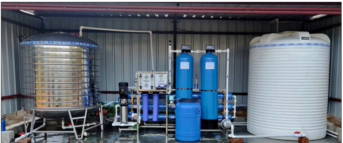
24 KLD Fully Automatic RO Water Treatment Plant
