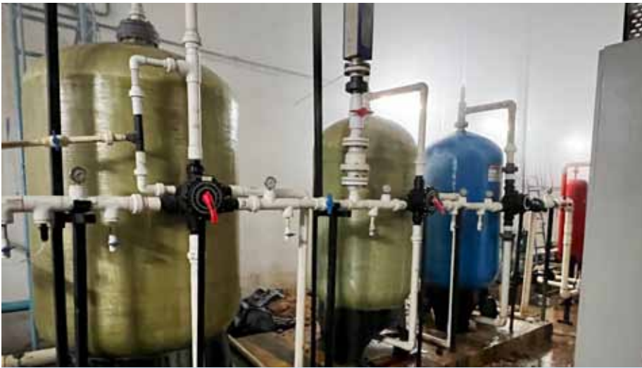
Pic 1.1-Existing Sand Filter System at Le-Meridien
